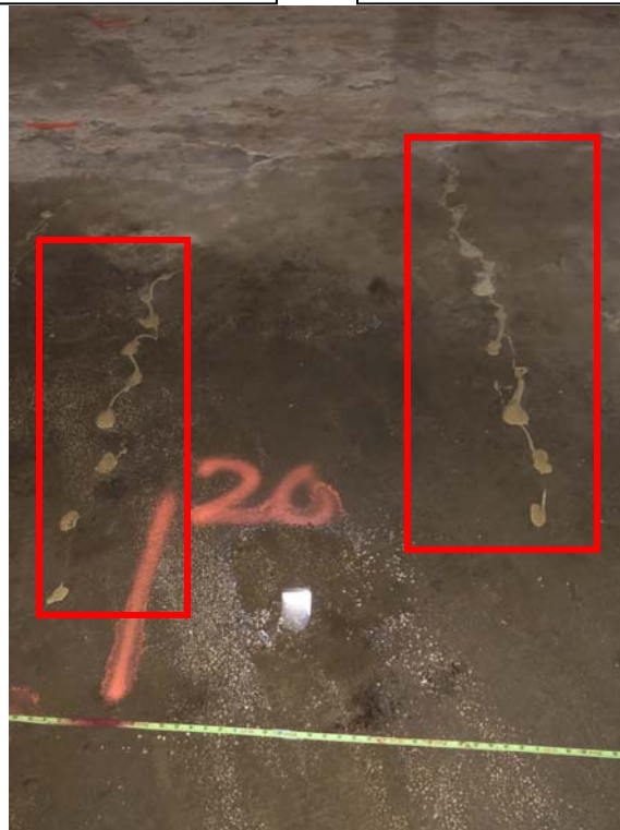
Site Picture 3 Showing Concrete Spalling Repairs on the Tank Floor Slab
