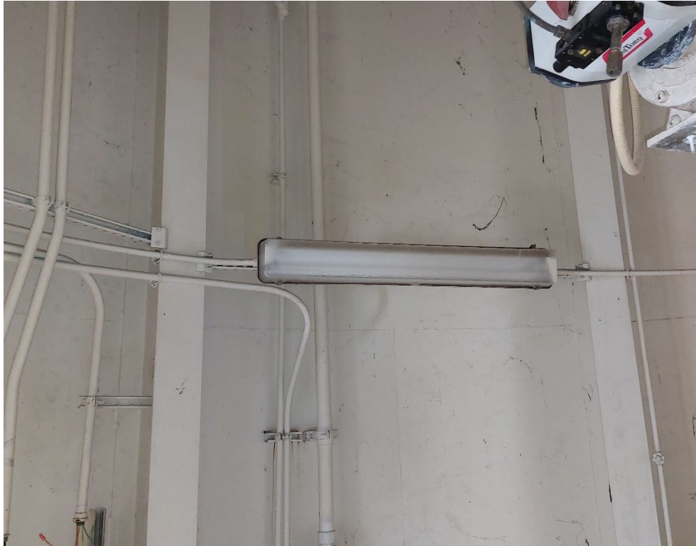
Photo 19 – Fluorescent light fixture with four-foot bulb
