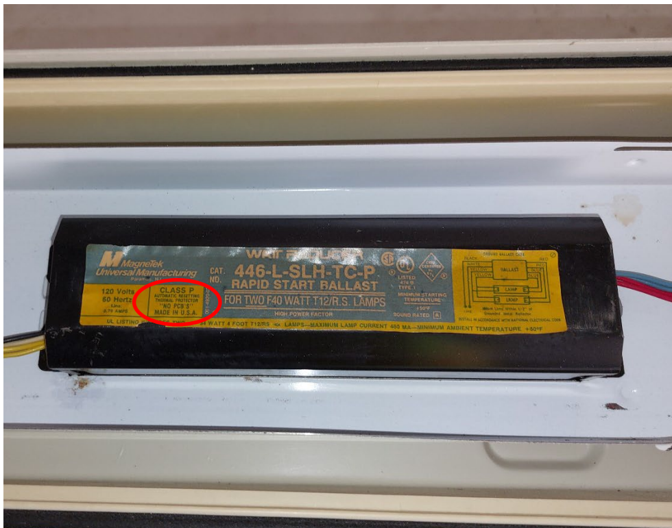
Photo 20 – “No PCB” labeling on all lighting ballasts observed
