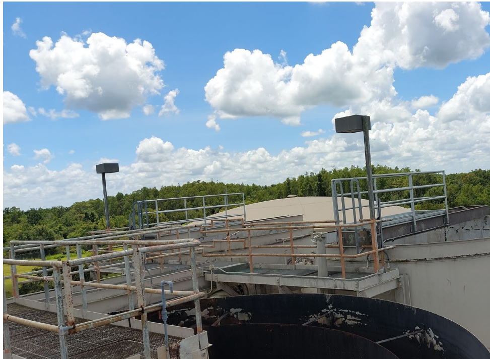
Photo 6 – LBP orange metal handrails on top of Structure 7
