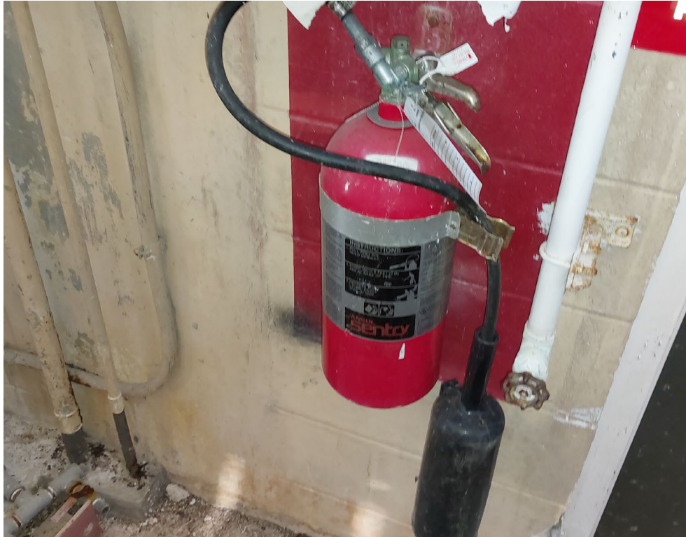
Photo 17 – wall mounted fire extinguisher
