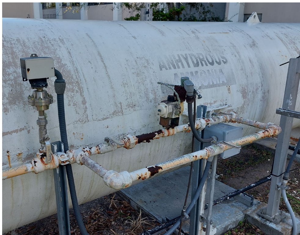
Photo 22 – “Chlorine Tank” labeled “Anhydrous Ammonia” in field
