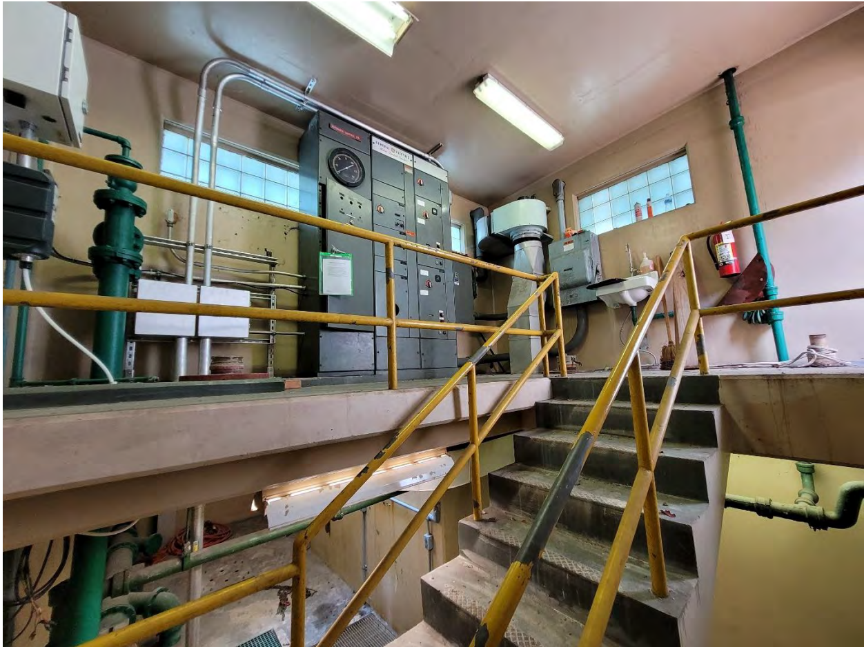
Pump Stat 183: Level 1
