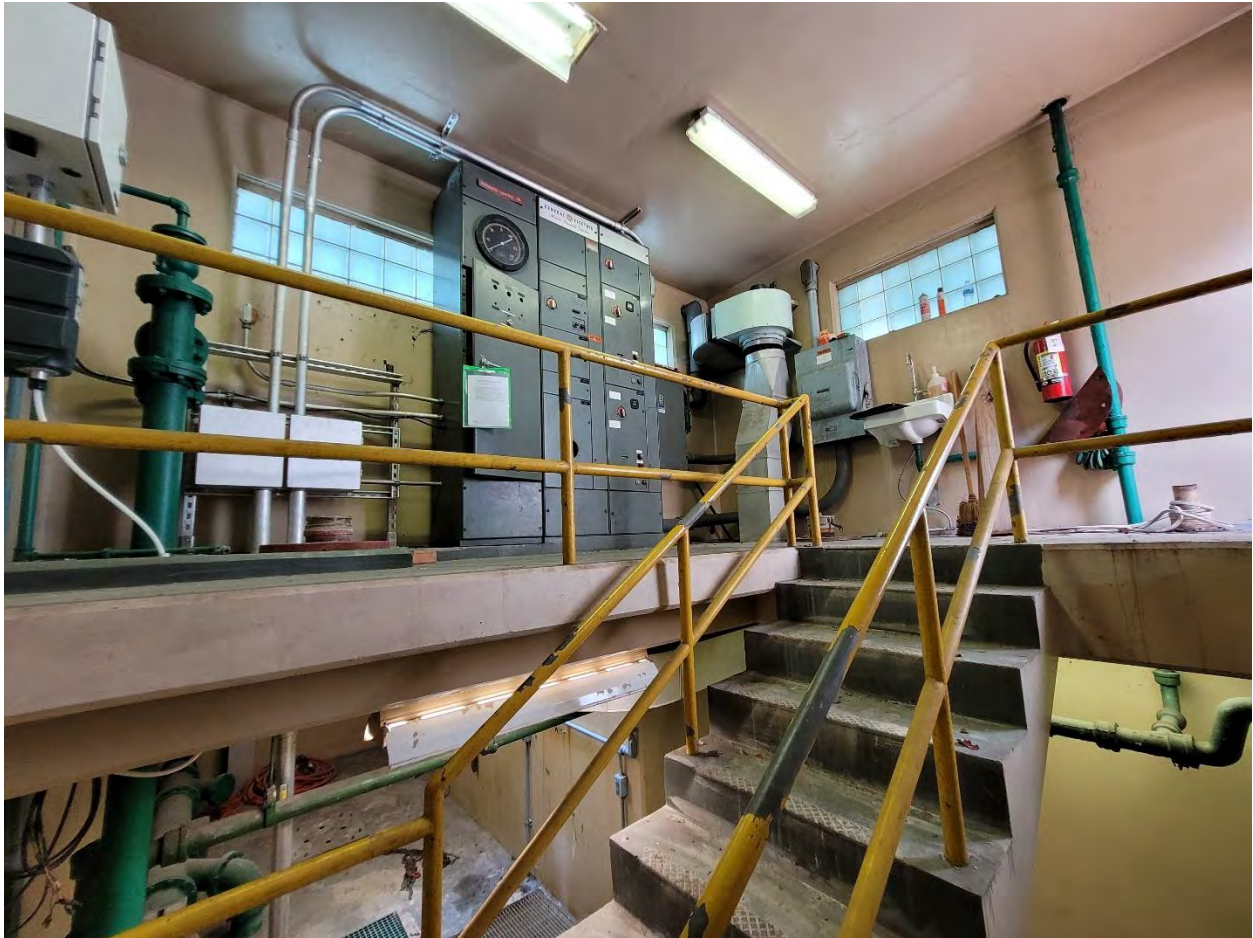
Pump Stat 183: Level 1
