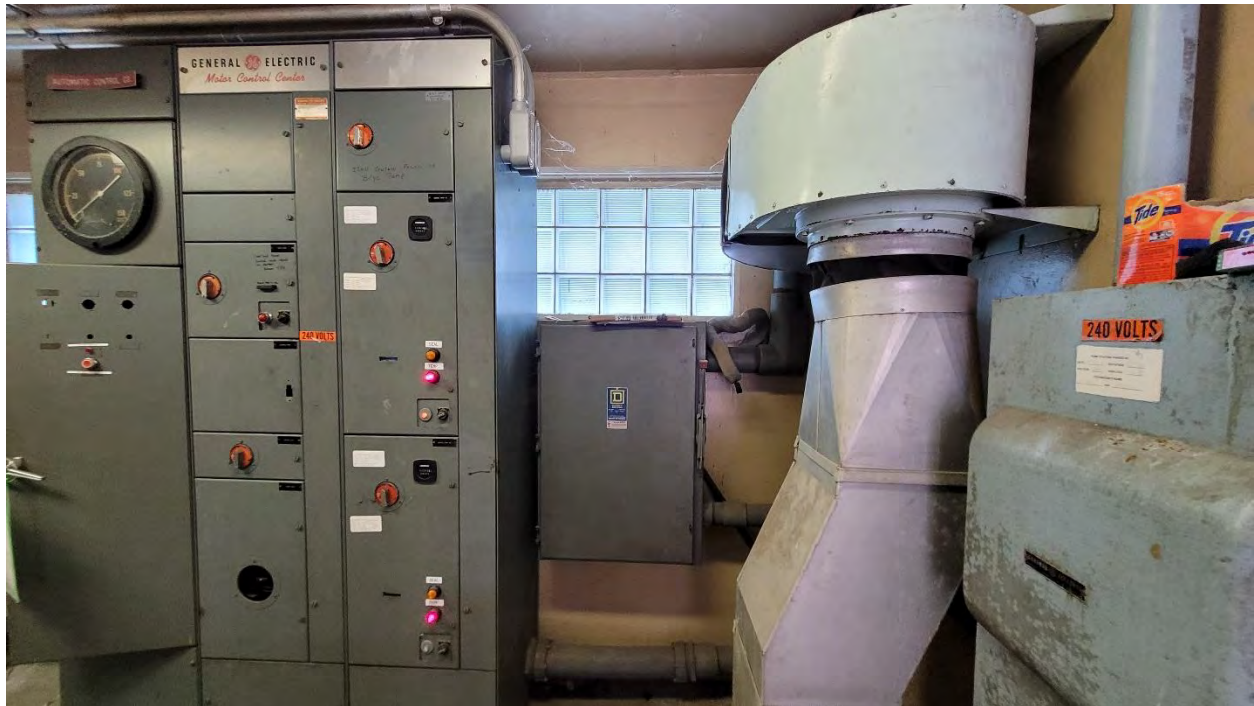
Electrical Panels and Ductwork should be sampled after the site is inactive
