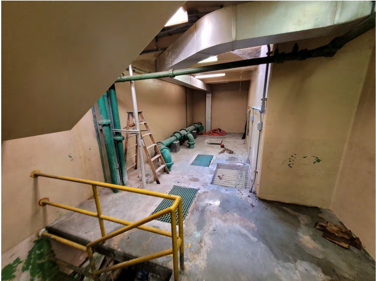
Pump Stat 183: Level 2
