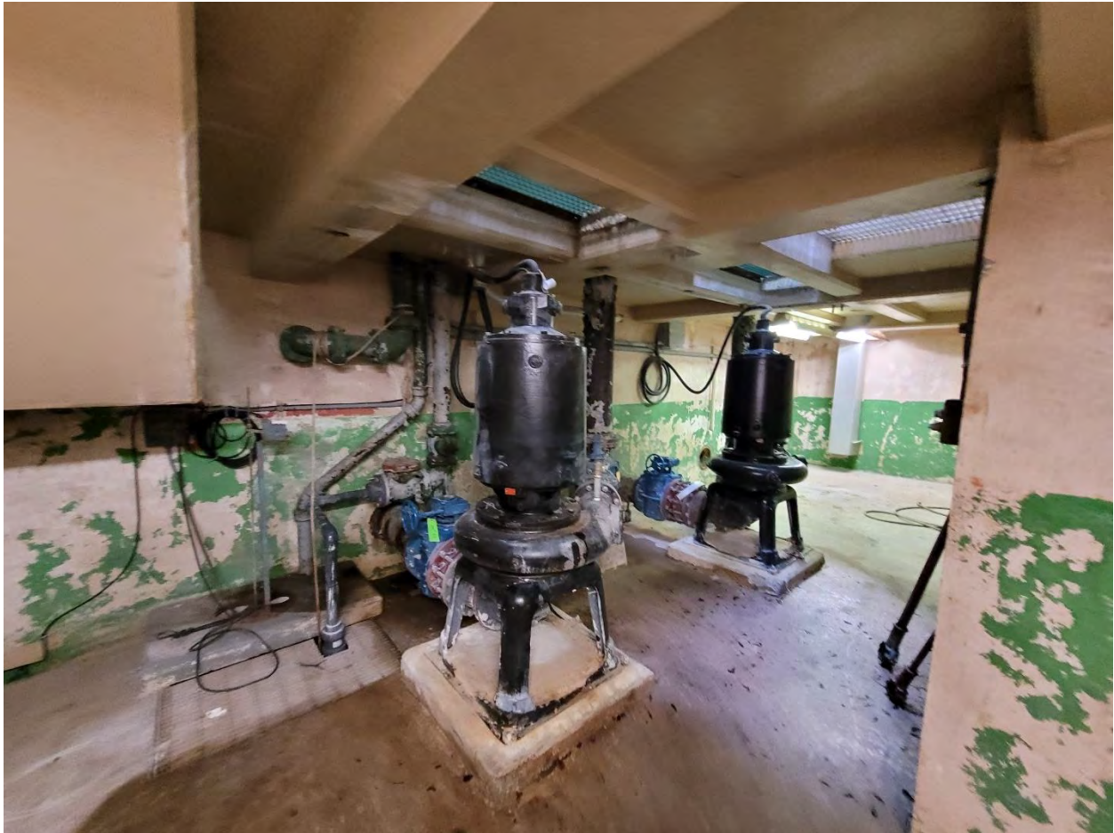
Pump Stat 183: Level 3
