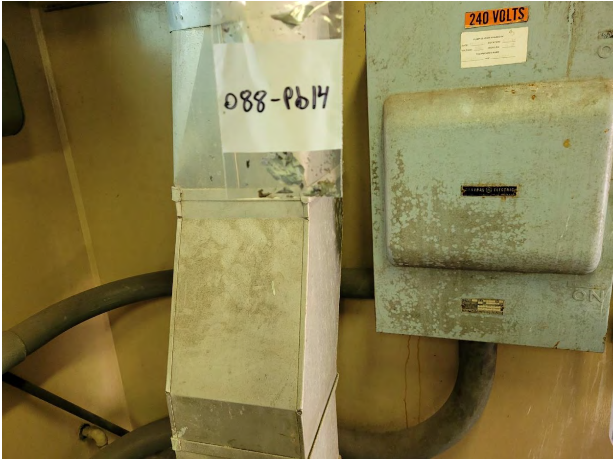
088-PB 14: Grey Paint on Metal Breaker Box [NLD]
