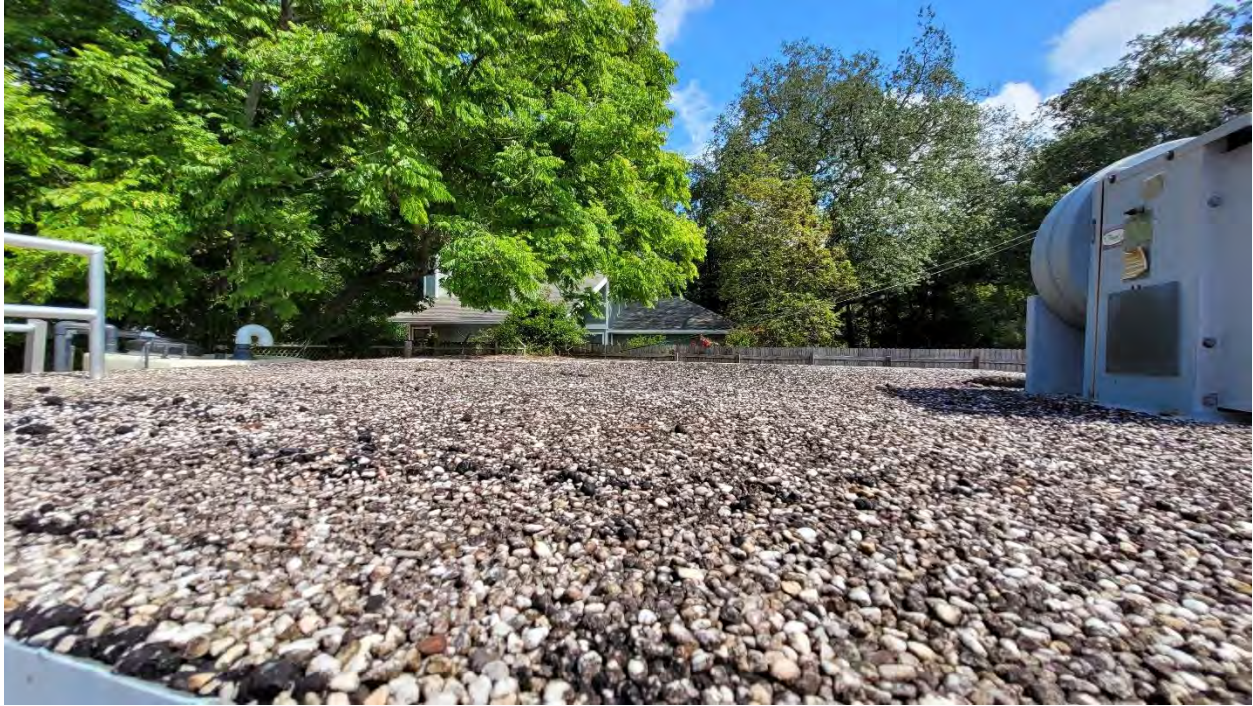
Roofing materials should be sampled after the site is inactive
