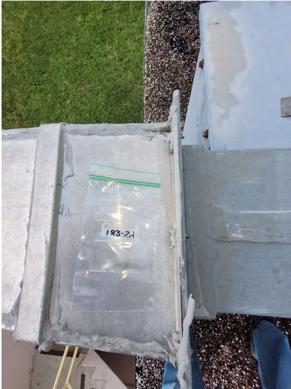
183-2A: HVAC Duct Mastic/Caulk [NAD]
