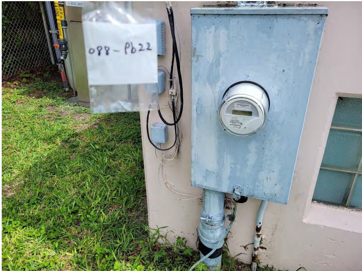
088-PB 22: Grey Paint on Electrical Box [NLD]
