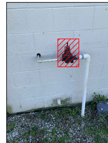
PHOTO 2 PRESSURE REGULATOR VALVE
