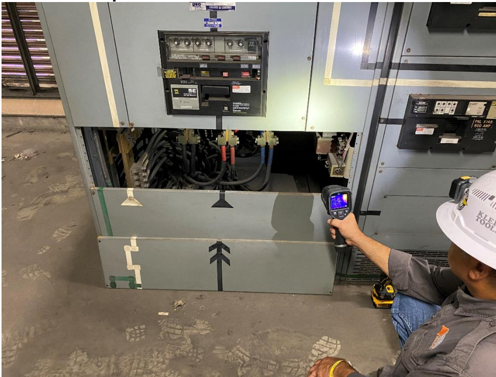
SWBT4A - IR Scan in progress
