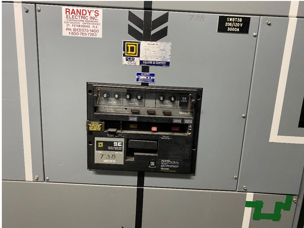
View of SWBT3B MAIN 3000a OCP with good condition rating plug.
