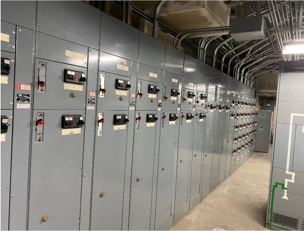
MCC – K11MCC-3- 50% to 65% of this MCC is not in operation.
