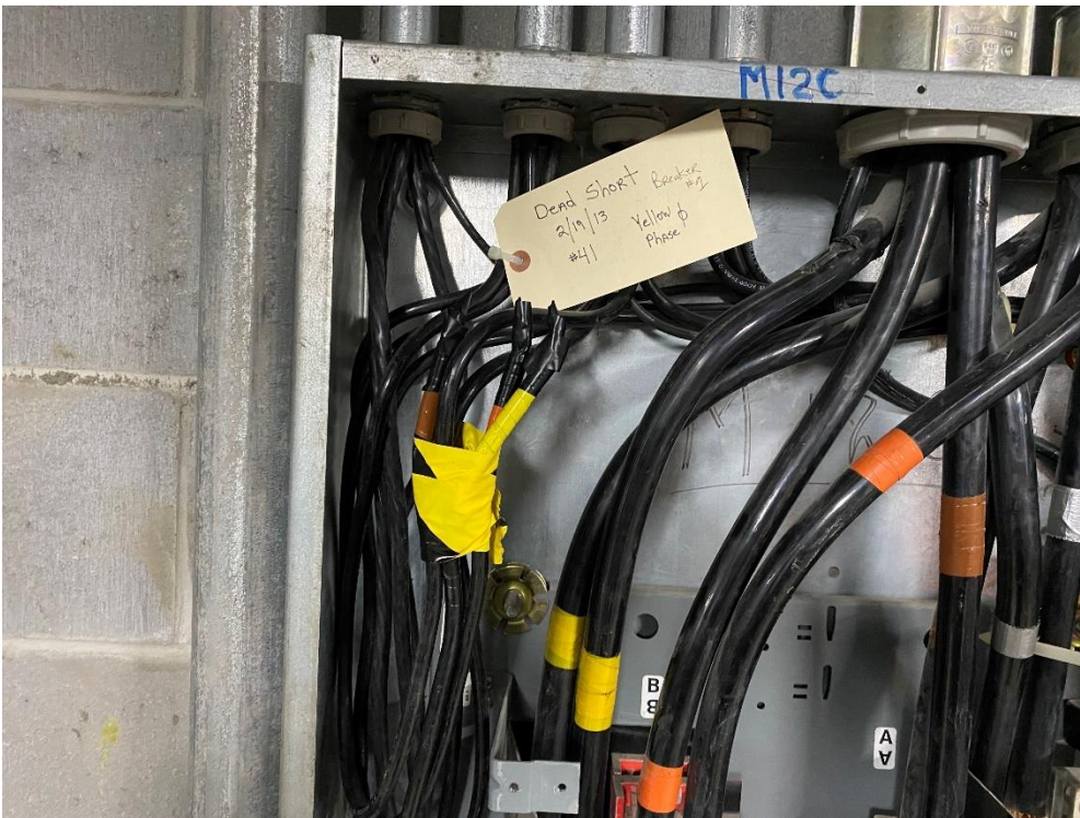
Panel M12C is in violation of the NEC. Owner needs to address ASAP.
