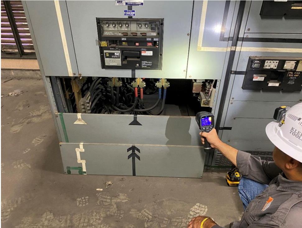
SWBT4A - IR Scan in progress
