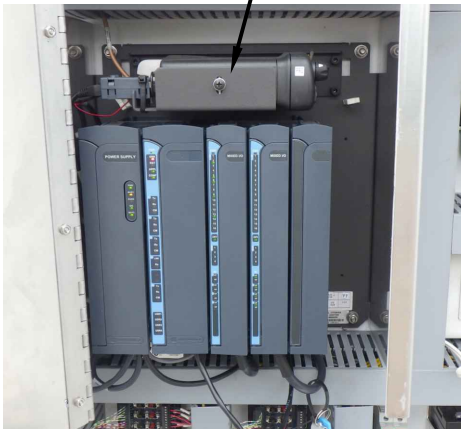
LAKE ECKLES PUMP STATION – CONTROL PANEL
