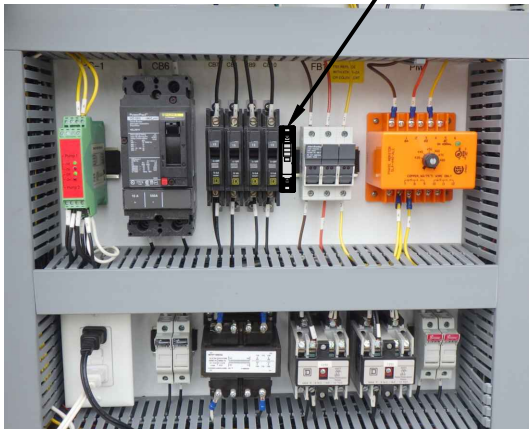
LAKE ECKLES PUMP STATION – CONTROL PANEL
