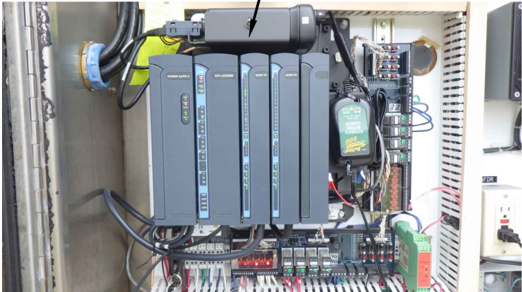
PENALTY LAKE PUMP STATION – CONTROL PANEL
