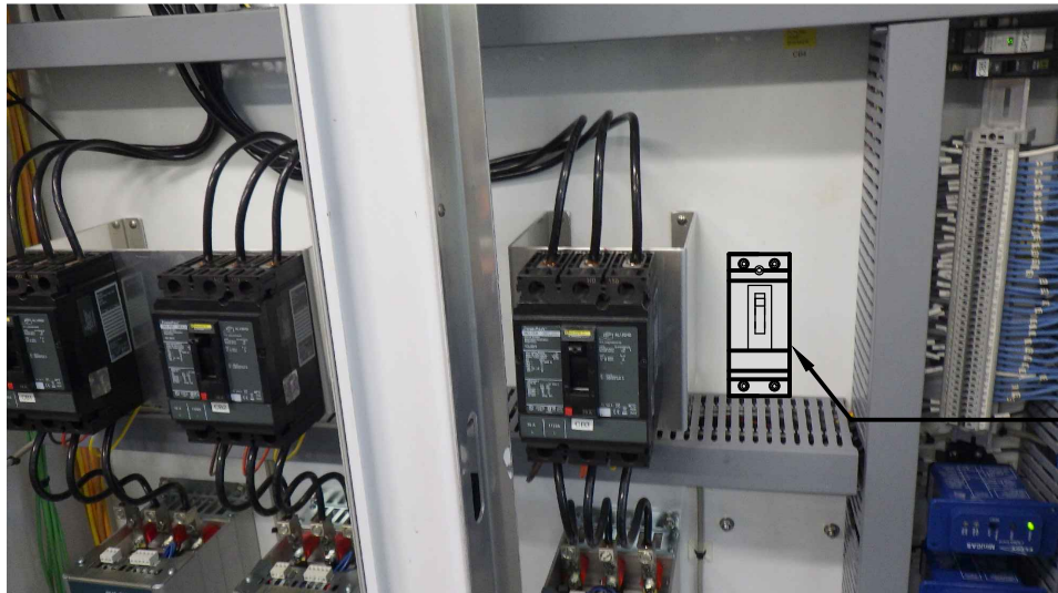
POINSETTIA PUMP STATION – MOTOR CONTROL PANEL
