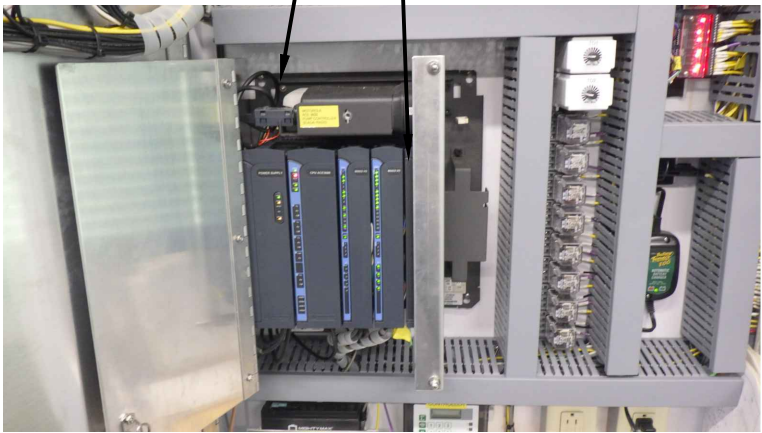
POINSETTIA PUMP STATION – PUMP CONTROL PANEL
