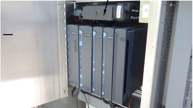
YORK STREET PUMP STATION – CONTROL PANEL
