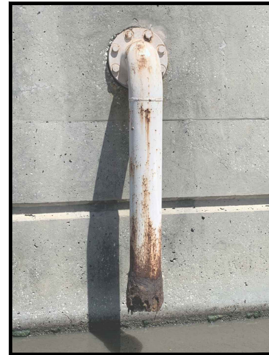
EXISTING SUMP PUMP DISCHARGE
