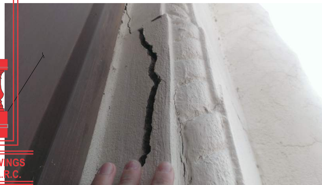
DAMAGE AT SIDE OF JAMB UNIT
