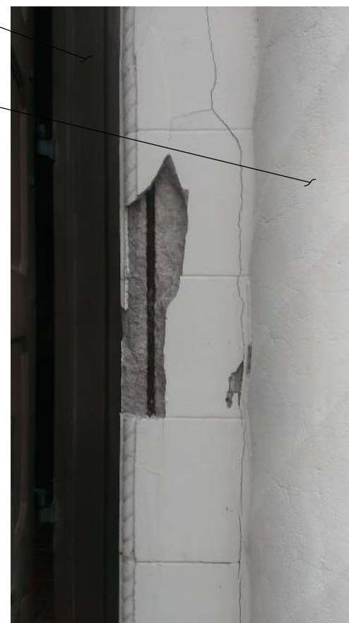
LOSS AT FACE OF JAMB UNIT
