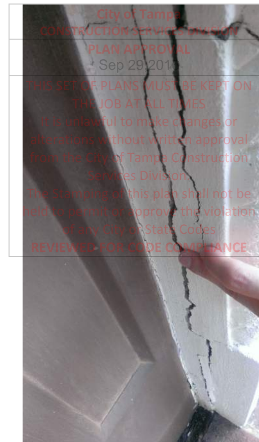
DAMAGE AT SIDE OF JAMB UNIT
