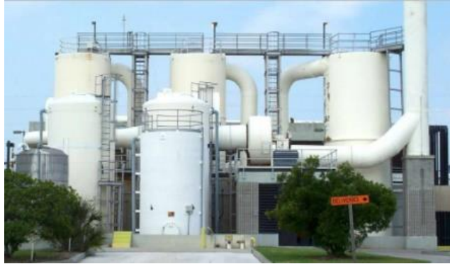
Source: City of Tampa Wastewater Department
