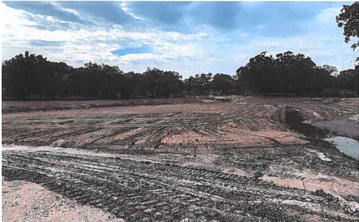
Expanded Stormwater Facility with Dry Bottom and Existing Drainage Creek
