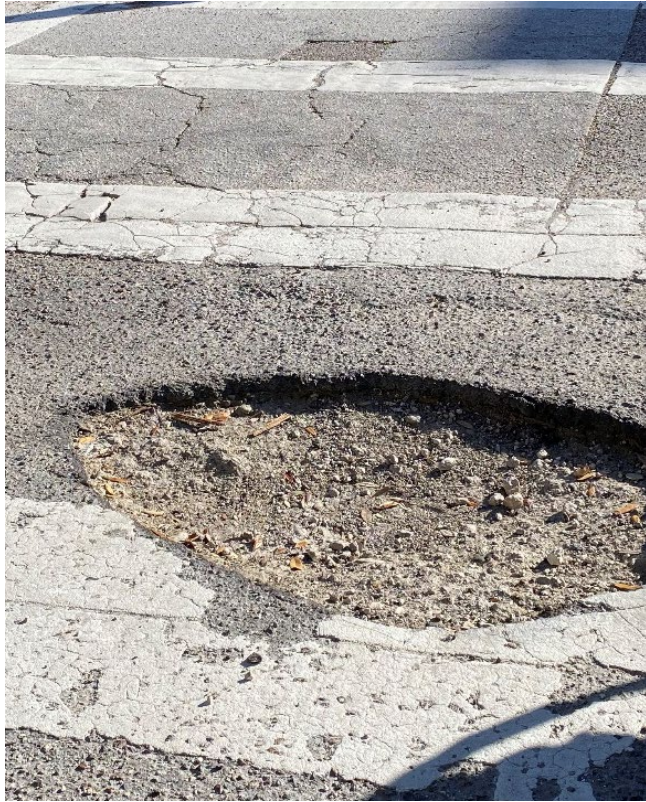
Paving - 40% of roads are in Poor Condition.
