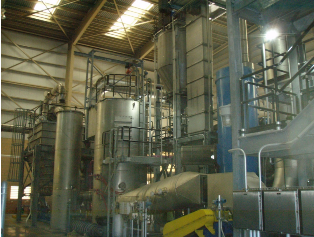
Figure 17.2-1: Existing 2 (Two) Andritz DD50 Rotary Drum Dryers at Hillsborough County's NWWRF
