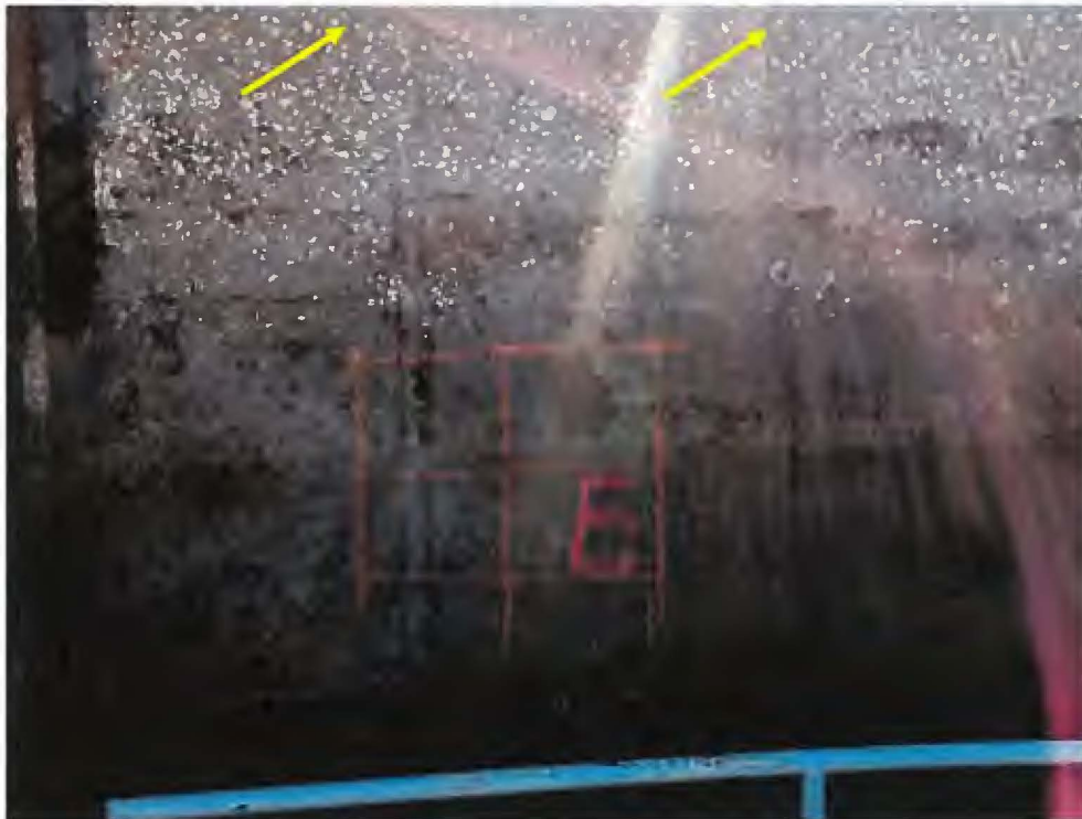
Photo 10 – East wall of tank with vertical cracks.
