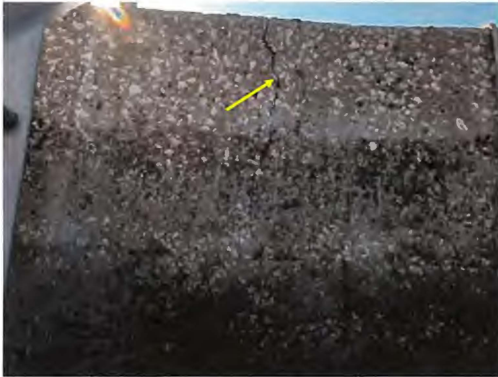
Photo 15 – South wall of tank with vertical cracks.
