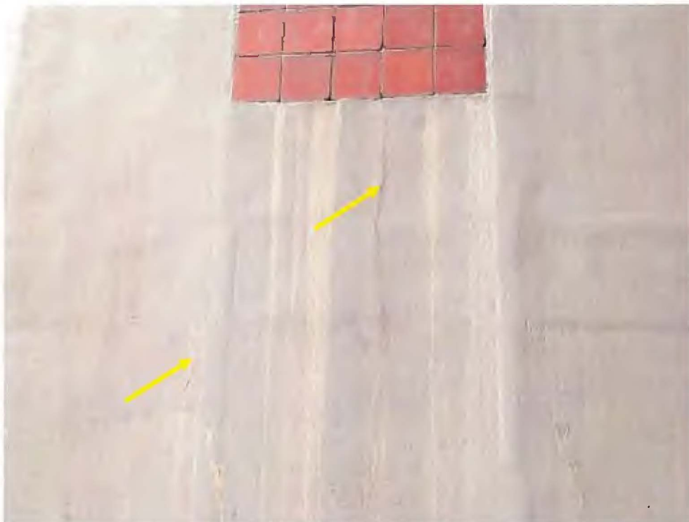
Photo 24 – East external wall of tank with vertical cracks.
