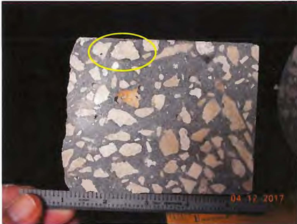
Photo 12 – Piece of coarse aggregate with partial ring/halo around it.
