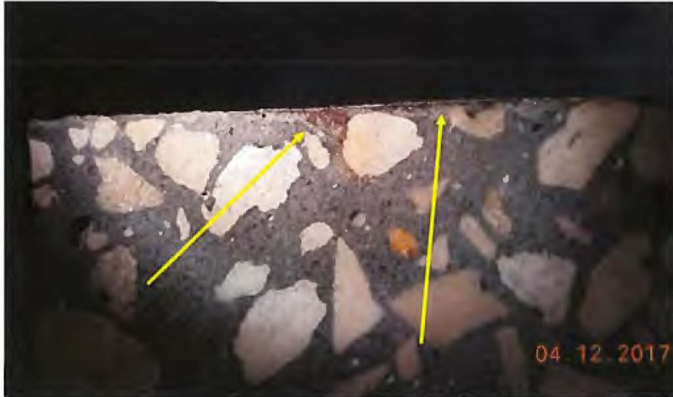
Photo 4 – Cross-sectional view of core surface. Note brown stained layer (Struvite crystals) at surface and deeper inclusion of stain.
