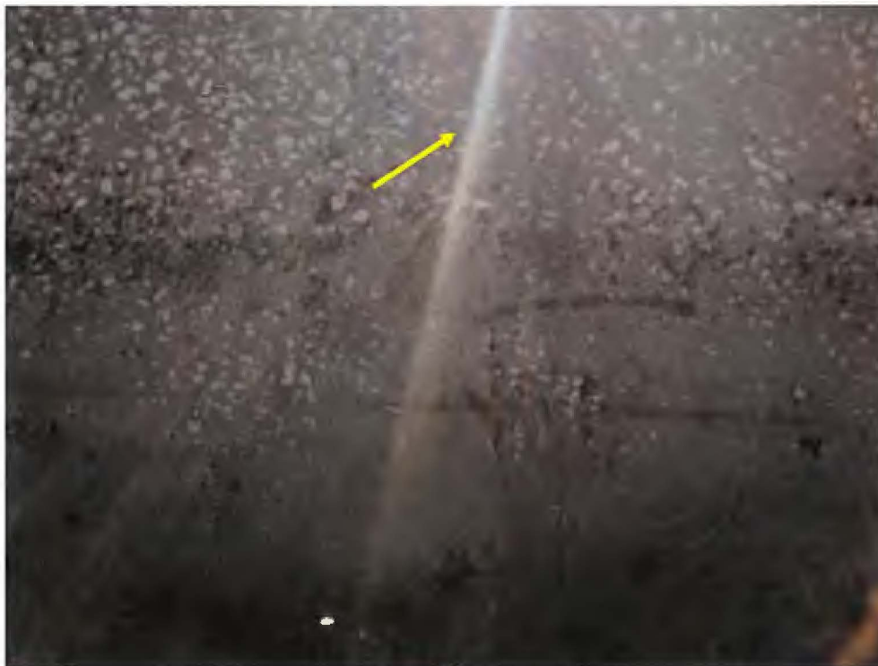
Photo 14 – Southeast wall of tank with vertical cracks.
