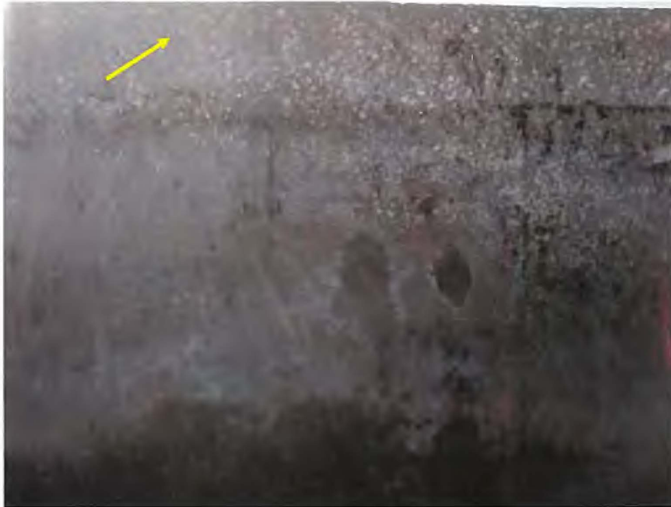
Photo 13 – Southeast wall of tank with vertical cracks.
