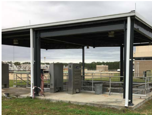
Figure 6.2-5: Similar Aqua Aerobic System Installation
