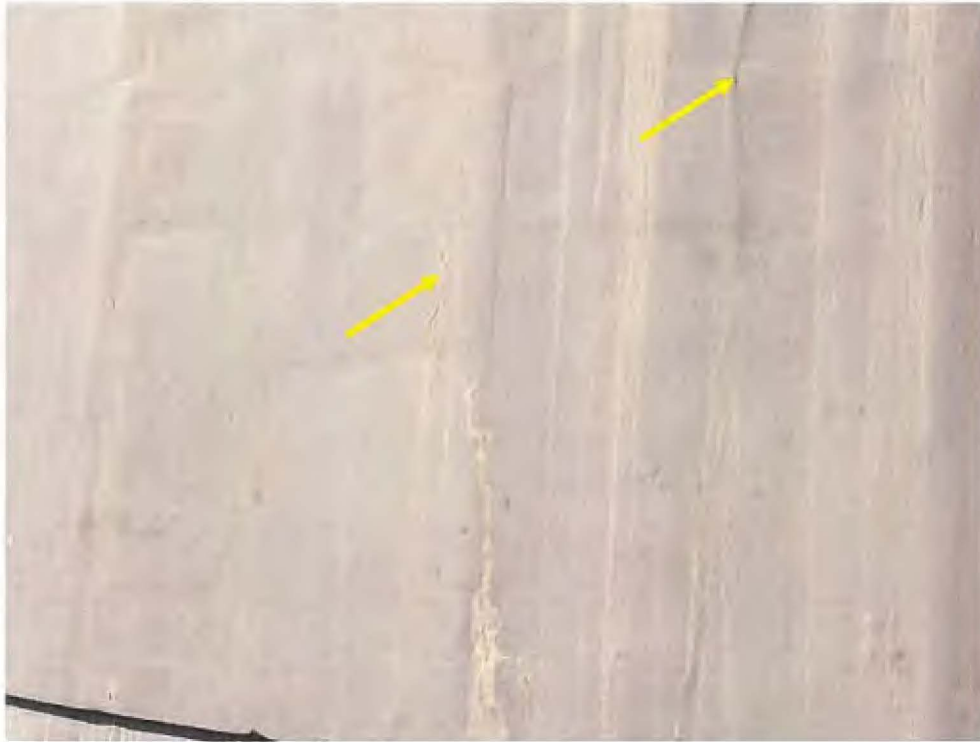
Photo 25 – South external wall of tank with vertical cracks.
