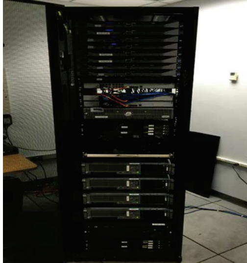
Figure 16.2-1: Administration Building Network Rack
