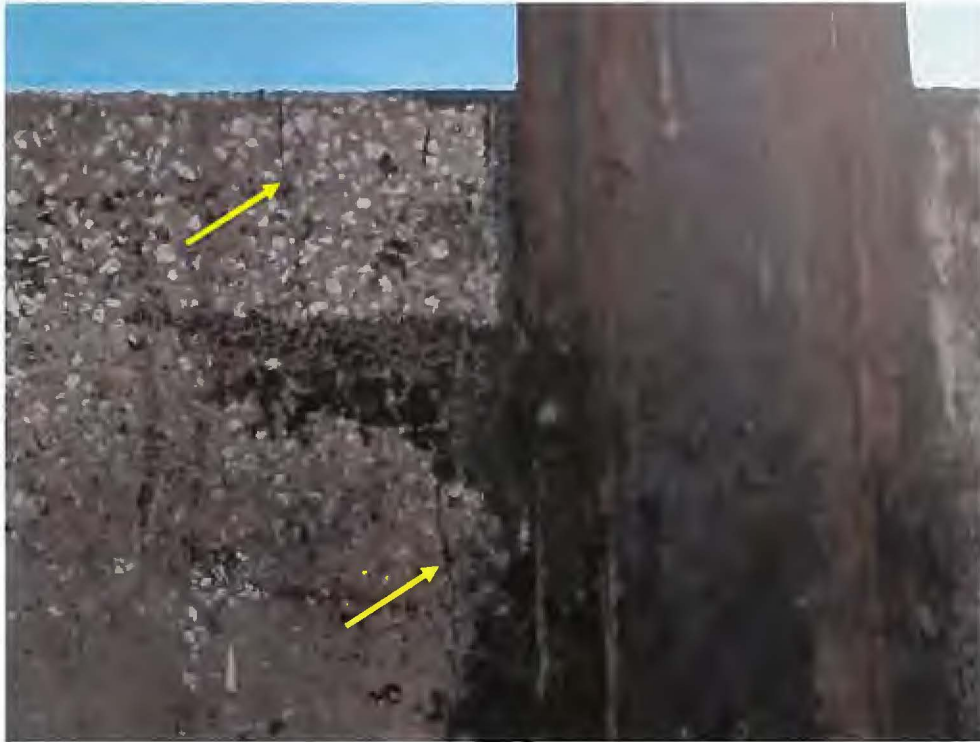
Photo 9 – East wall of tank with vertical cracks.
