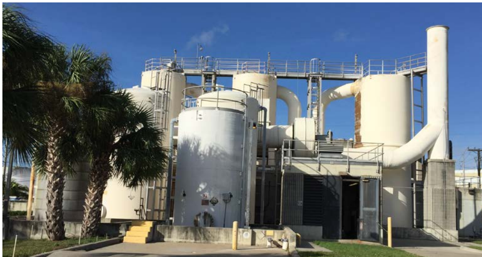
Figure 5.2-1: Photo of Existing Odor Control System
