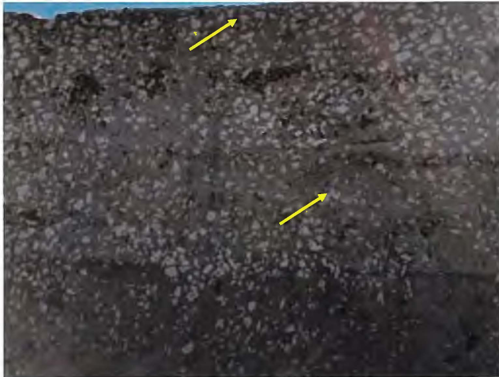
Photo 11 – East wall of tank with vertical cracks.
