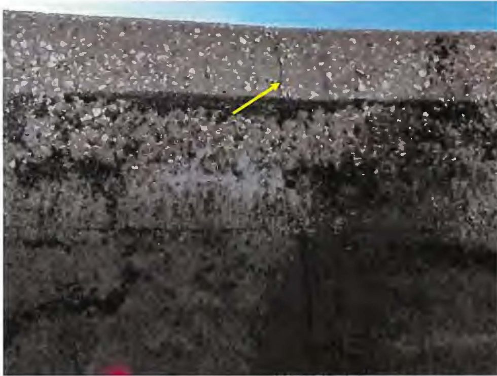
Photo 19 – West wall of tank with vertical cracks.
