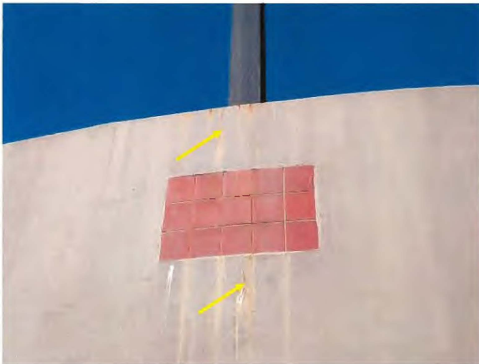
Photo 26 – West external wall of tank with vertical cracks.
