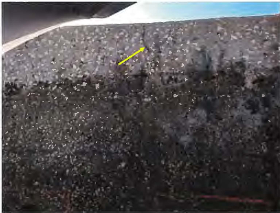
Photo 18 – West wall of tank with vertical cracks.
