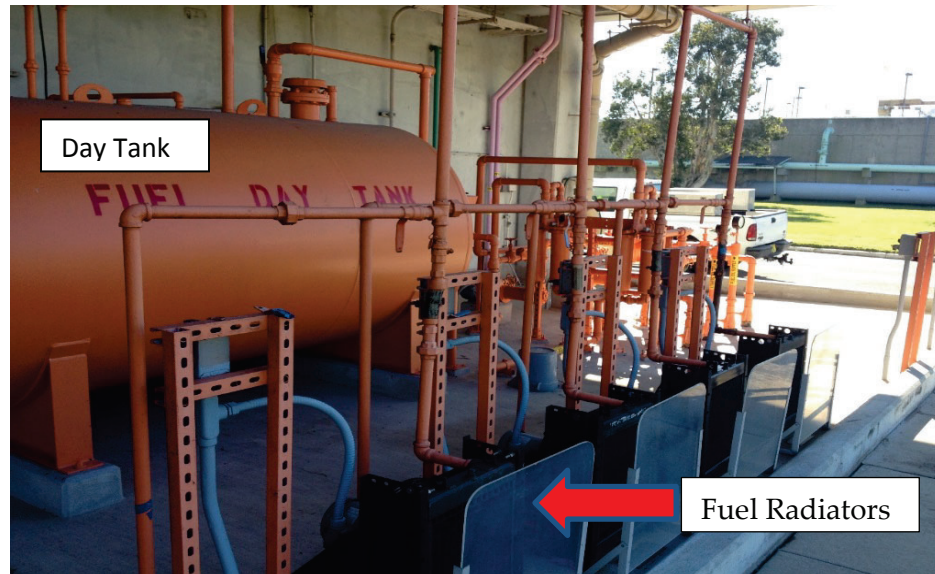
Figure 15.3-1 – Day Tank Fuel System and Fuel Radiators
