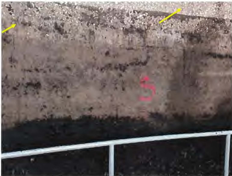
Photo 16 – South wall of tank with vertical cracks.
