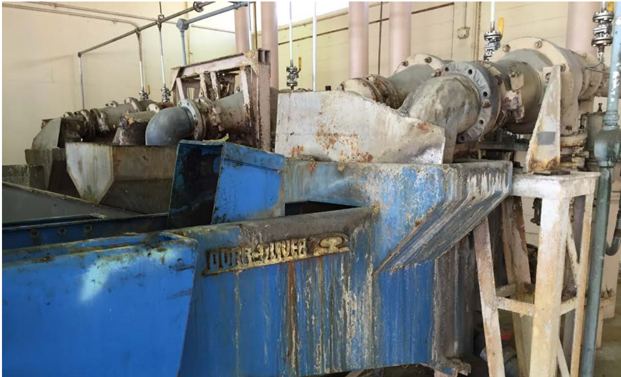
Figure 5.4-1: Photo of Existing Grit Removal Equipment
