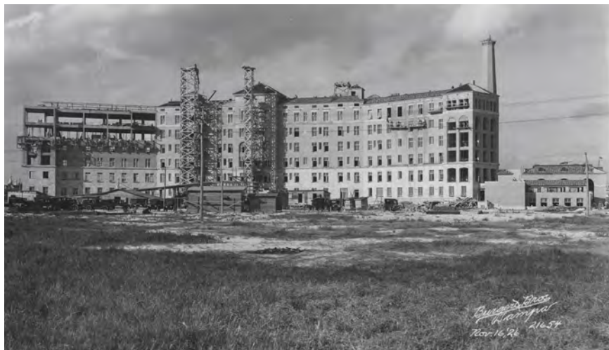
Construction of Tampa Municipal Hospital (now Tampa General Hospital) on Davis Islands, November 16, 1926.
