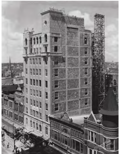
Tampa Theatre building on Franklin Street (700 block), front and side facades under construction on August 30, 1926.
