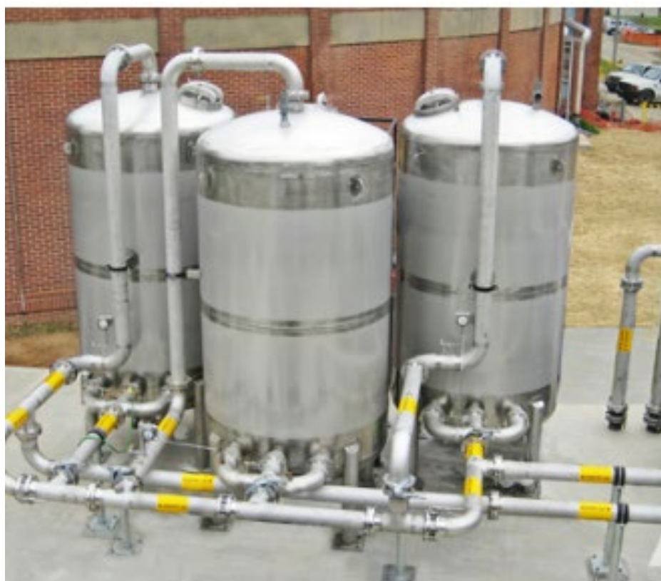
Figure 3-6: Non-Regenerative Siloxane Removal System (Unison)
