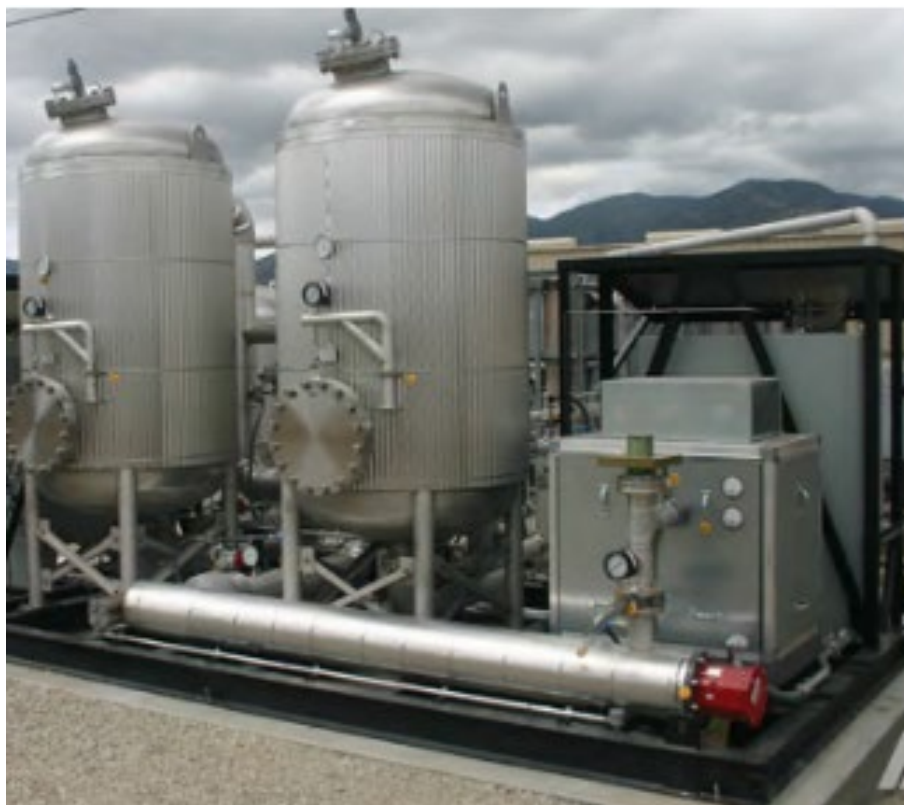
Figure 3-7: “Twin-Tower” Regenerative Siloxane Removal System (Unison)
