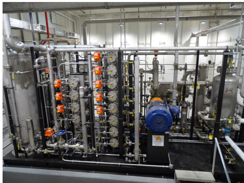
RNG Upgrading Membranes
