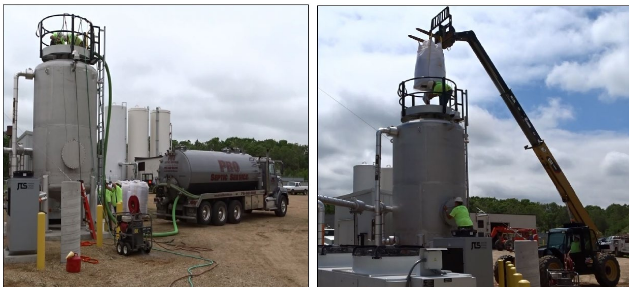
Figure 4-5: Left, exhausted media being removed from H 2 S polisher. Right, vessel being filled with new media. (Unison Solutions)
