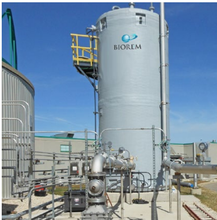
Figure 3-5: BTF System (Biorem)
