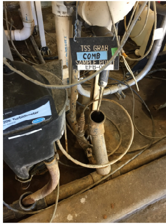
Figure 2-12: Final Effluent Grab Sample Location
