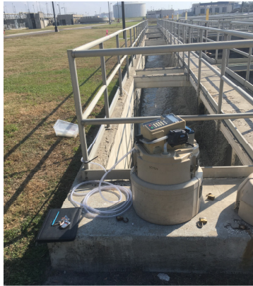
Figure 2-2: Primary Effluent Composite Sampler
