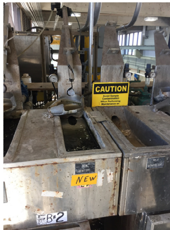
Figure 2-11: Denitrification Filter Effluent Grab Sample Location
