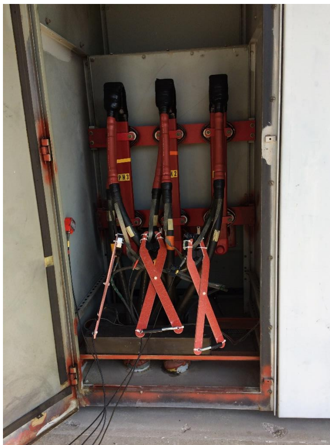
Photo 1: Example of HFCT and TEV sensor placement in the cable cubicle.
