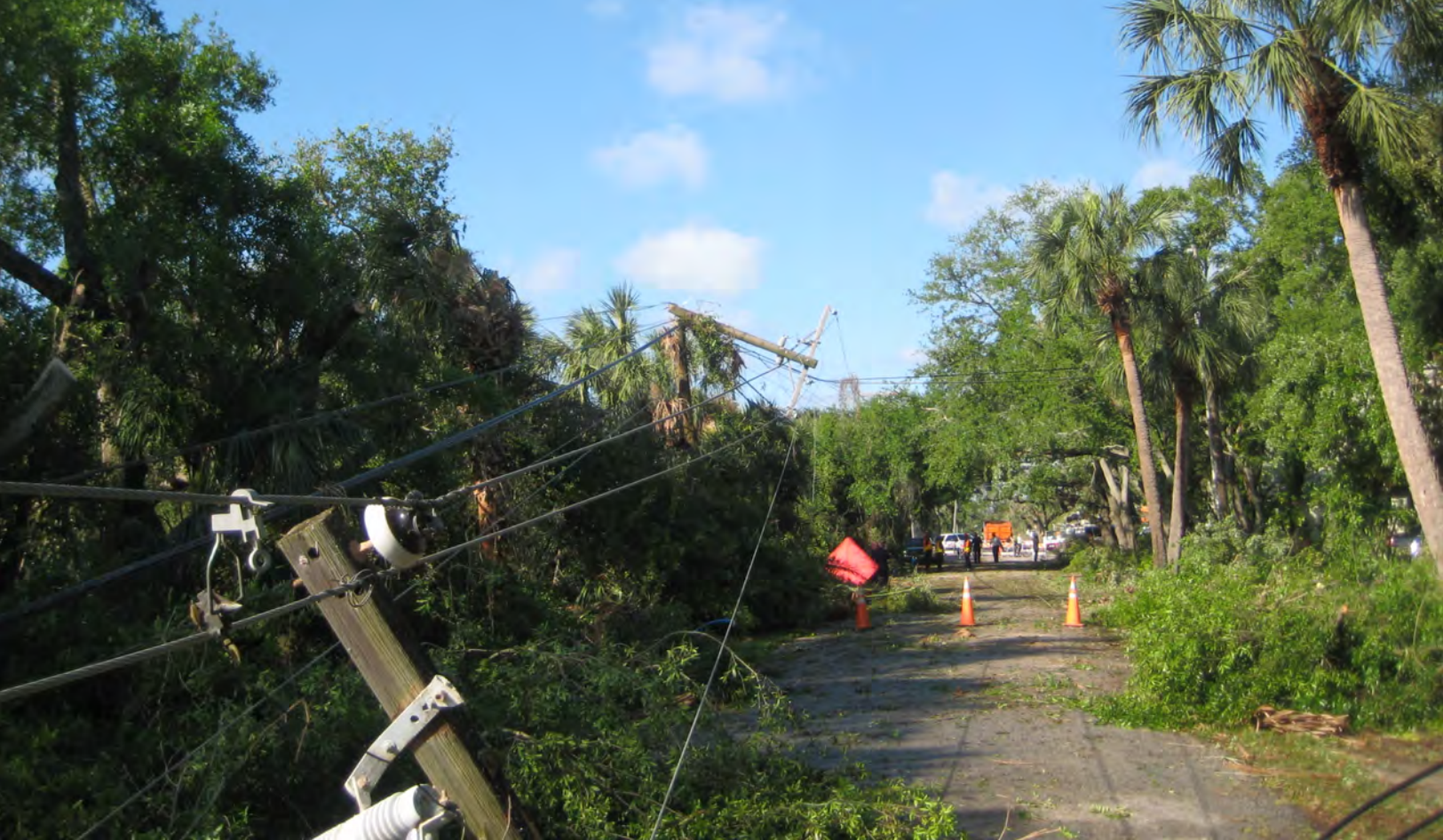
Damage from tornado that touched-down in April 2011 along Interbay Boulevard in Tampa.
